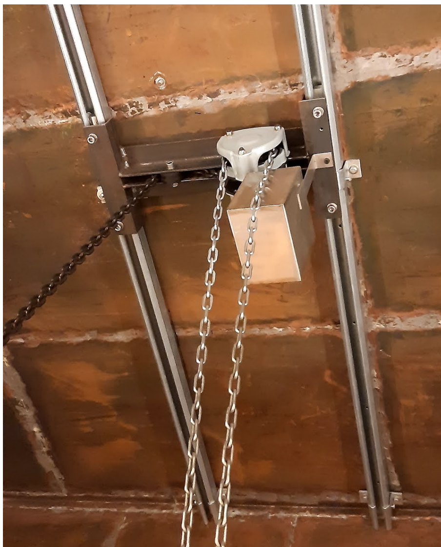
Figure 5.18: An image showing the crane used for moving the insert in and out of the cryostat.
